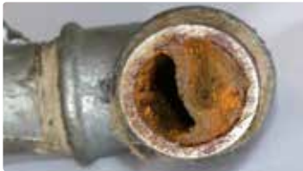
Pipe with scale deposits
